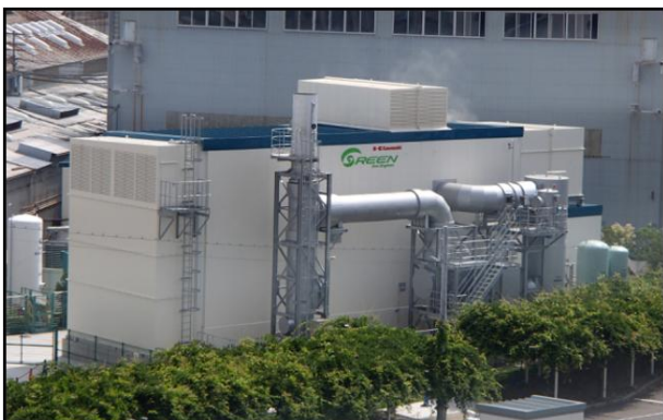
Mazda considers introducing a gas cogeneration system (Photo: Kawasaki Heavy Industries, Ltd. Kobe Plant Power Center No. 3)
