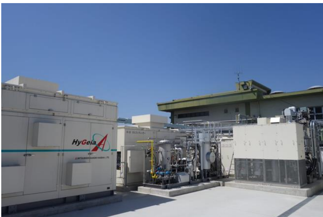
Fukuoka City hydrogen production facility
